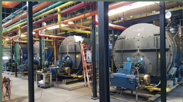
Iola Powerhouse & Cogeneration Facility
