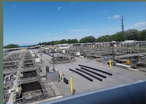
Monroe County Water Resource Recovery Facility
