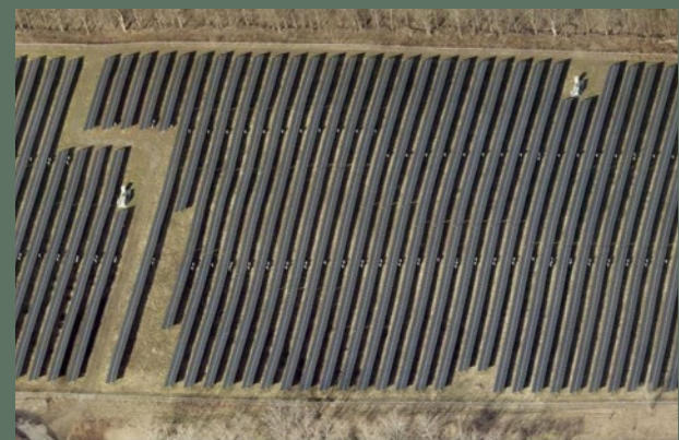
Monroe County Solar Farm
