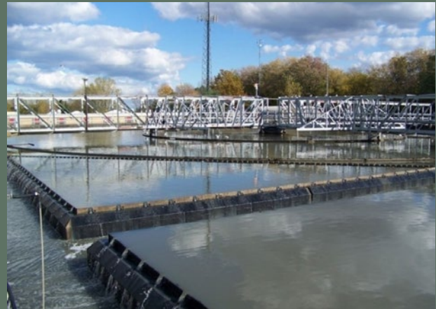
Monroe County Water Resource Recovery Facility
